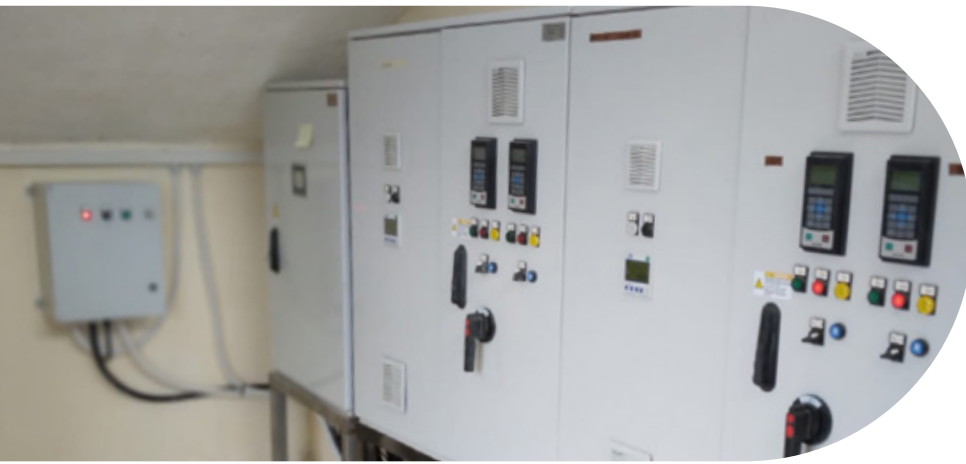
FIG Bahar ic-Caghaq Wasteserve .09 Pumping Station
