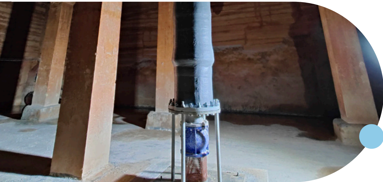
FIG Temporary and .08 Contingency Pumps
