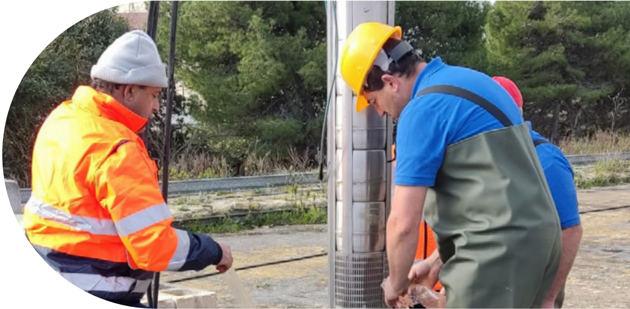
FIG Temporary and .07 Contingency Pumps
