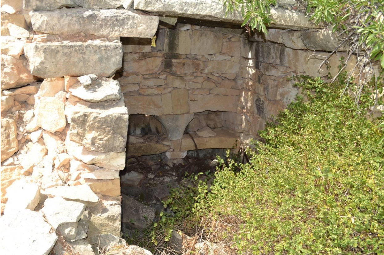
Figure 46. Internal view of the partly collapsed apiary (Photo credit David Cadona)
