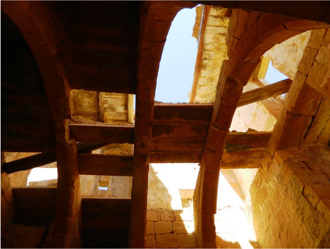
Figure 38. Id-Dar ta' Pultu internal collapsed ceilings (Photo credit Ruben Abela)
