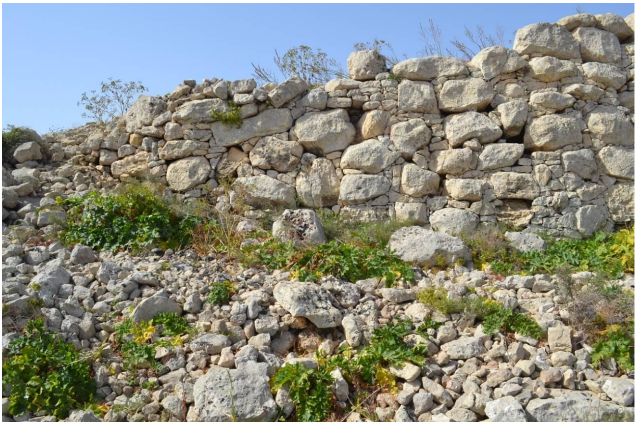
Figure 29. Part of the original wall together with signs of the restoration conducted at the turn of the century. On the left side of the photograph an area where a collapse has occurred is also visible (Photograph credit Josef Caruana)
