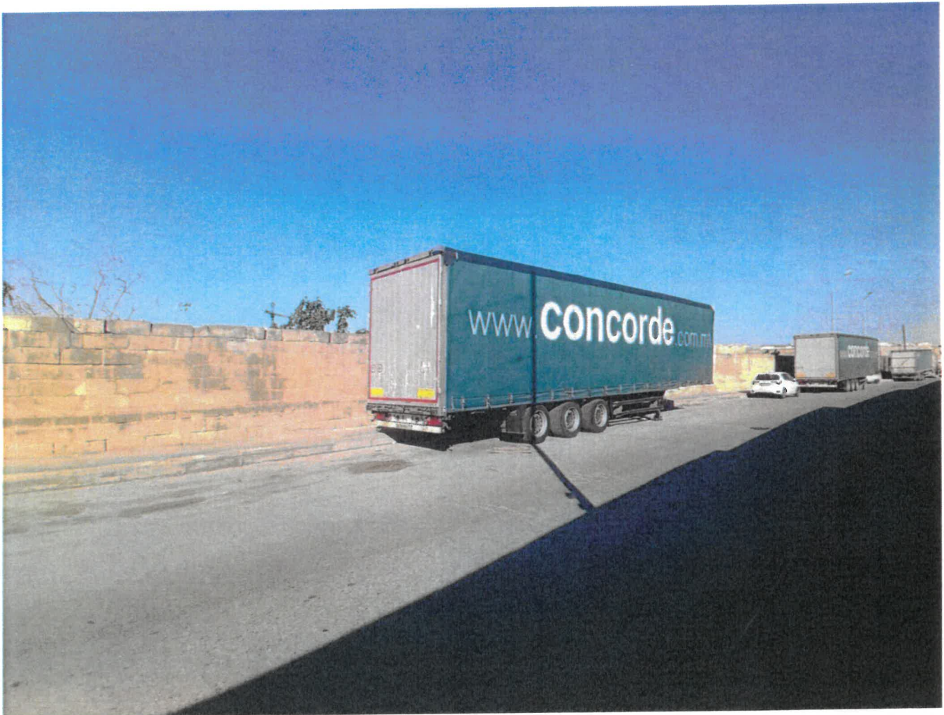
Photo 2: Photo showing the boundary wall of the land in question from the other road.
