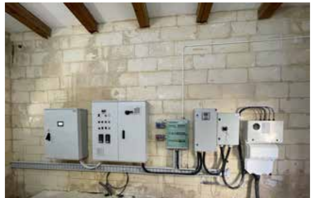
Fig. 14 New electrical control equipment at Għajn Dwieli WWPS
