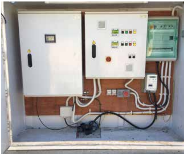
Fig. 13 New electrical control equipment at Xwieki Santa Katerina WWPS
