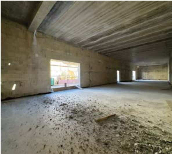
Figure 87 New blower room and storage facilities at Ta' Barkat WWTP
