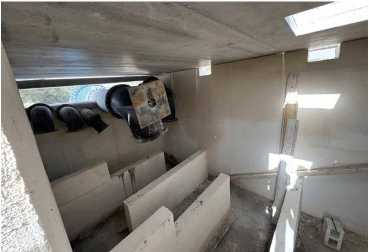
Figure 43 Ta' Qali reservoirs network restructuring and new blending weir room
