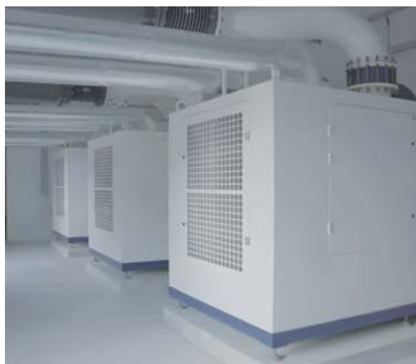
Figure 49 The new aeration system
