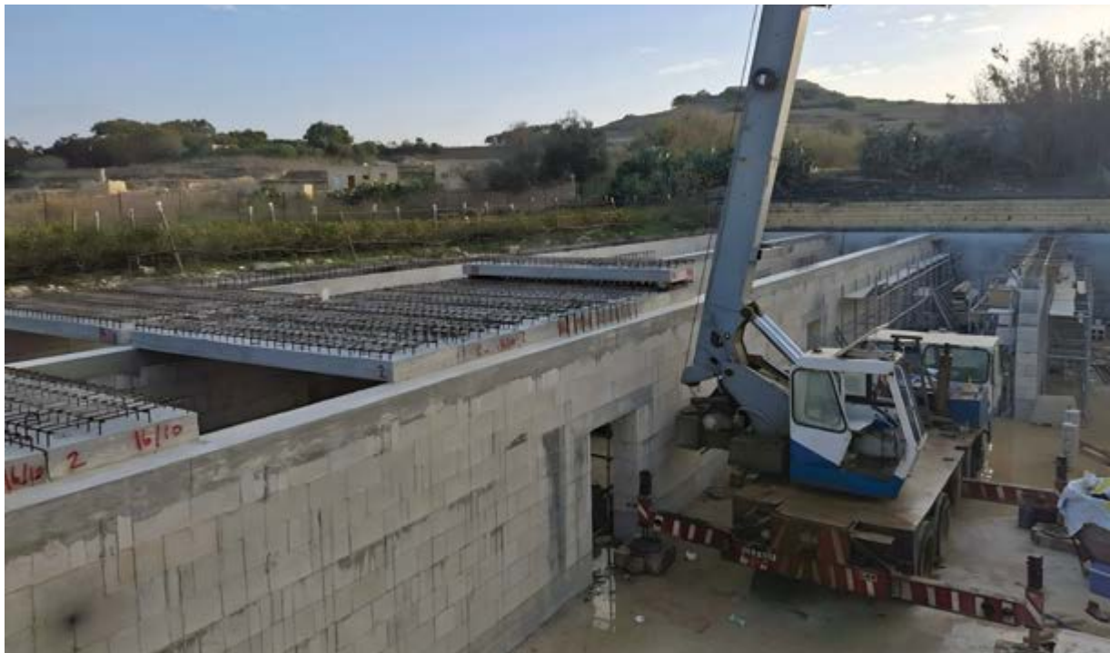
Figure 33 New second-class water reservoir constructed in Gozo
