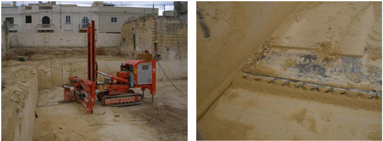
Figure 4-2: New stone cutting plant in operation Close-up of cutting blade
